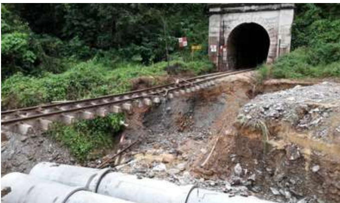
RESTORATION OF TRACK AND SLOPE STABILIZATION, TRACK REHABILITATION AND ASSOCIATED WORKS DUE TO MAJOR FLOOD BETWEEN GUA MUSANG AND TUMPAT RAILWAY STATION, KELANTAN PACKAGE C – EAST COAST (CIVIL WORKS)
